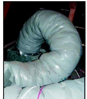
Bad duct installation prevents good air flow
